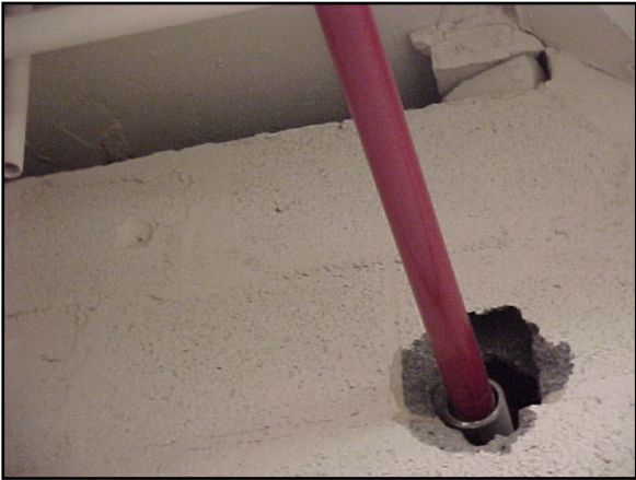
Figure 1: Pipe poking through a wall
