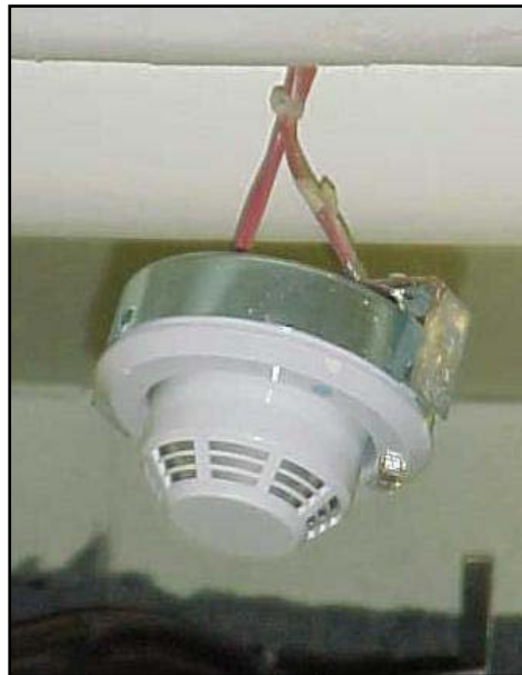
Figure 4: Loose smoke detector
