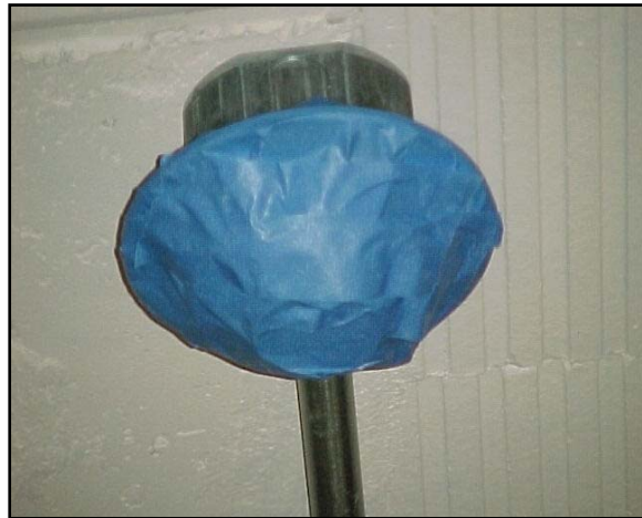
Figure 3: Smoke detector covered with tape
