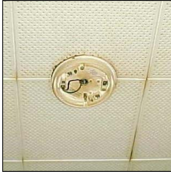
Figure 5: Missing smoke detector
