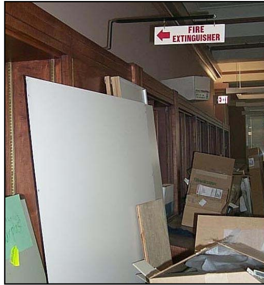
Figure 4: Inaccessible fire extinguisher
