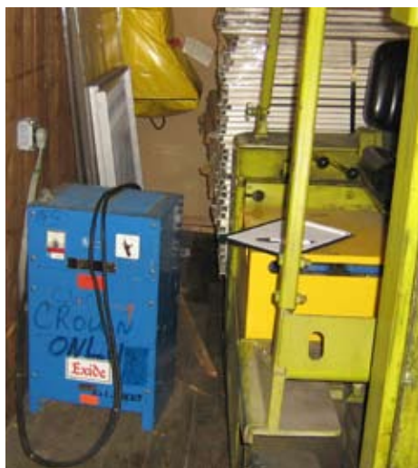
Figure 1: Battery Charging Station for a Forklift with Blocked Non-plumbed Eye Wash with Inspection Tag Attached
