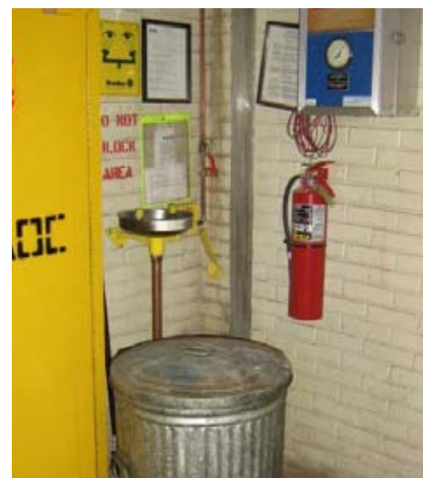
Figure 2: Obstructed Access to an Eye Wash
