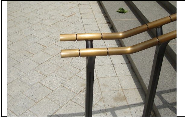
Hazard: Protruding handrails create projection hazard not compliant with 29 CFR § 1910.23(e)(5)(i), 2000 NFPA 101 7.2.2.4.5, ANSI/ASSE A1264.1-2007 Section 5.8 and ASTM E 985-00 Section 4.3.2.
