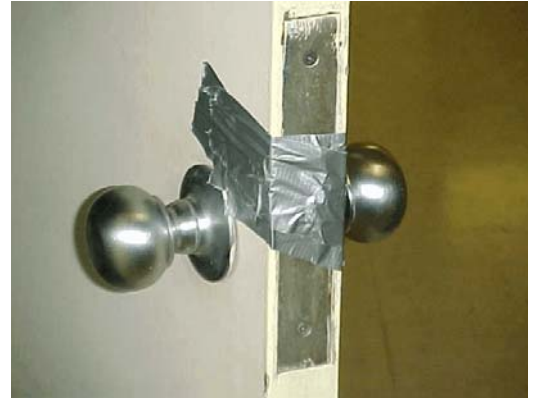
Fire door latch improperly taped to hold the door open
