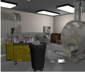
Figure 4: Improper Storage in Air Handling Room
