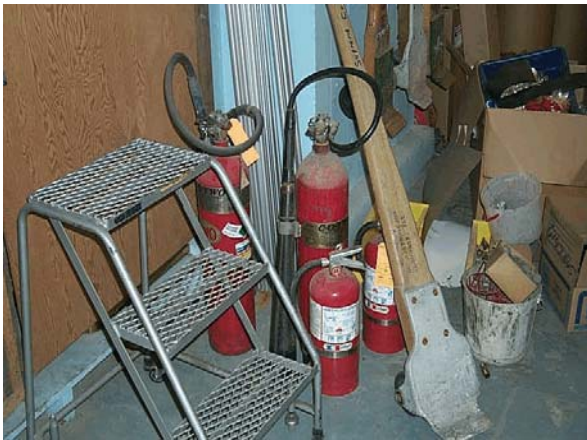
Figure 2 Carbon dioxide extinguisher not properly secured and placed.
