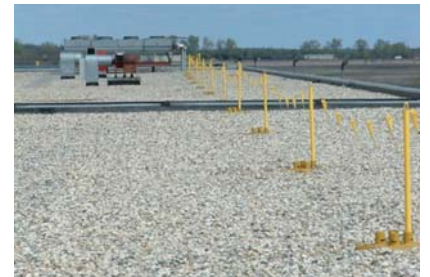
Fig. 7: Warning lines keep workers aware of and away from roof edges.
