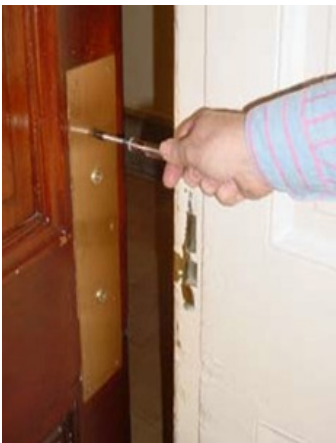
Image 1: The force required to open this door is too great.
