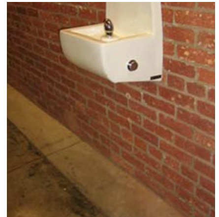
Image 2: Leading edge on this water fountain is too high: more than 27 inches above the floor.
