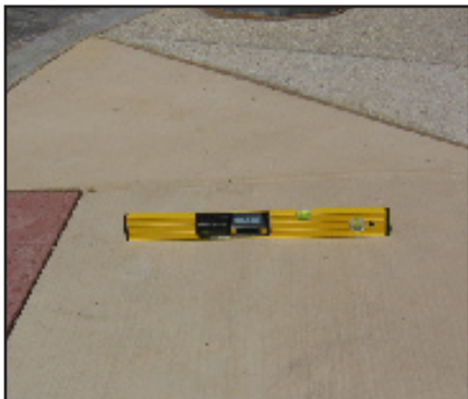
Figure 2: Non-compliant newly installed sidewalk curb cut
