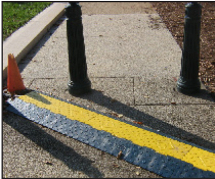
Figure 1: Non-compliant temporary sidewalk ramp
