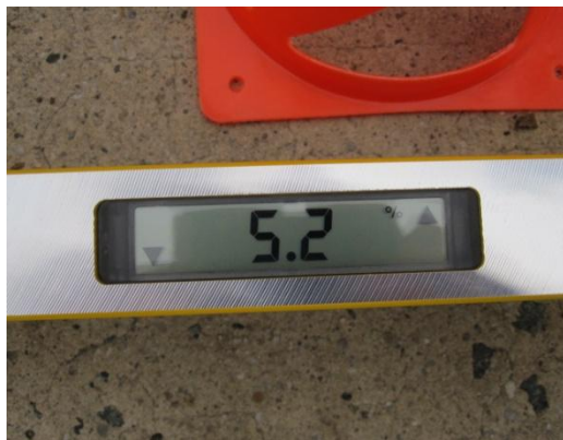
Curb Ramp 40 Has a Cross Slope of 5.2%
