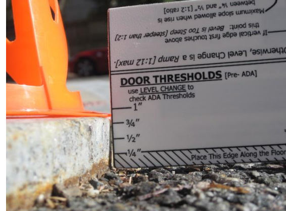
Transition Too High (Curb Ramp 27)
