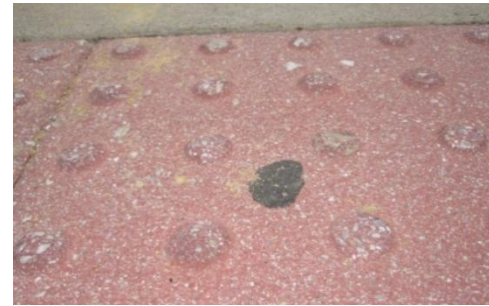
Deteriorated Detectable Warning (Curb Ramp 39)
