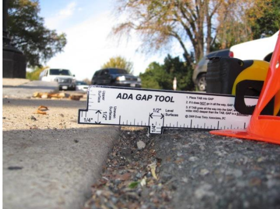
Slab Joint Too Wide & Too Deep (Curb Ramp 20)
