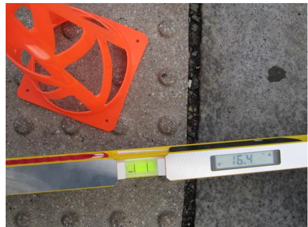
Curb Ramp 14 has a Running Slope of 16.4%
