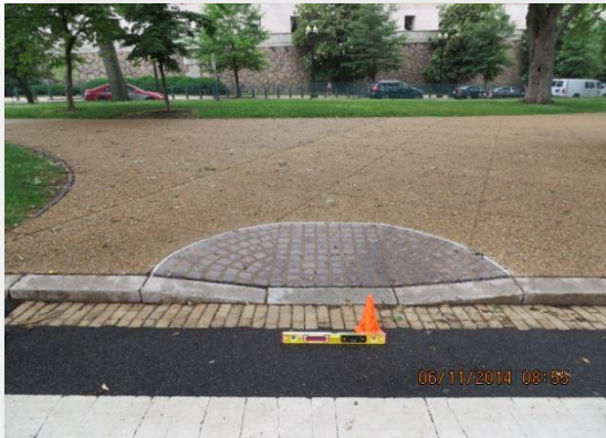
Figure 2. A Capitol grounds curb ramp with a cross slope that is too steep.
