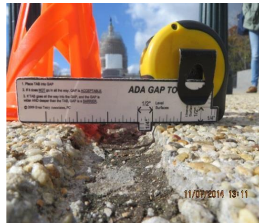
Figure 5. A wide gap within the expansion joint of a sidewalk on the east side of the Capitol.
