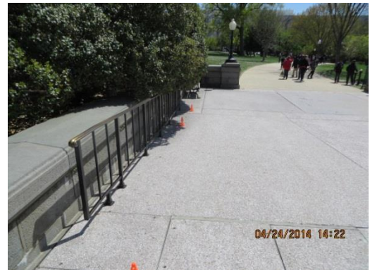
Figure 7. A ramp on the Capitol grounds with foliage obstructions to the handrails.
