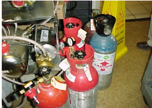
Unsecured Compressed Gas Cylinders
