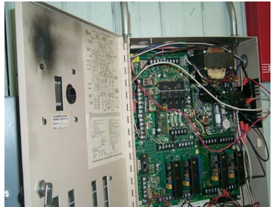
Fire Alarm Electrical Panel Requiring Repairs
