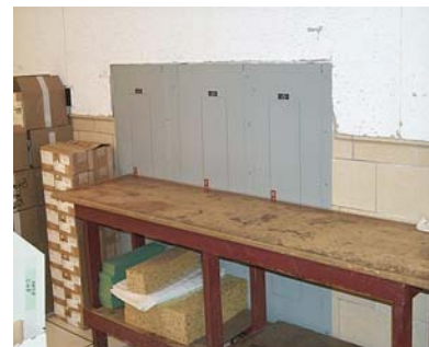
Blocked Electrical Cabinets Prevent Access in Case of an Emergency
