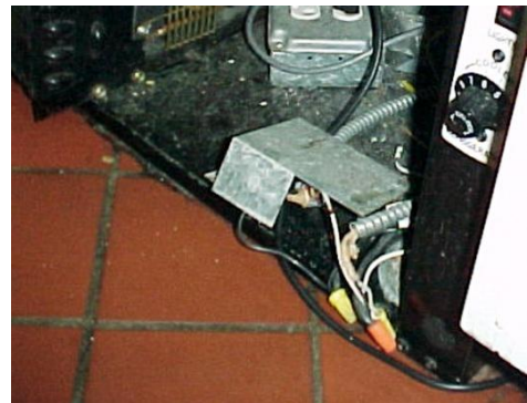
Picture 1: Open Electrical Box.
