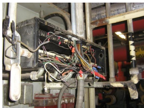
Picture 1: Back Electrical Cover Missing On Control Panel
