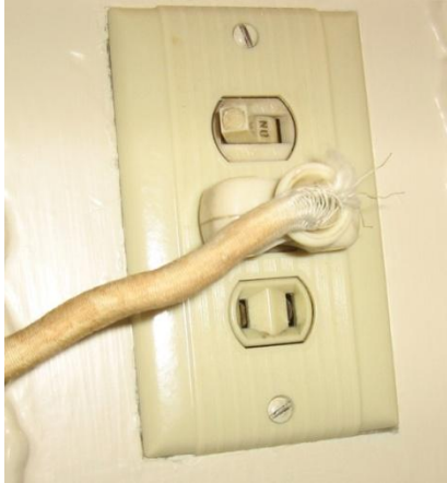
Picture 1: Two Prong Electrical Outlets Must Be Replaced With 3 Prong Outlets
