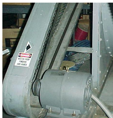
Picture 2: Inadequate Guard Over V-belt & Pulley
