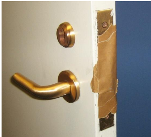
Picture 2: Fire Door Latch is Taped Open
