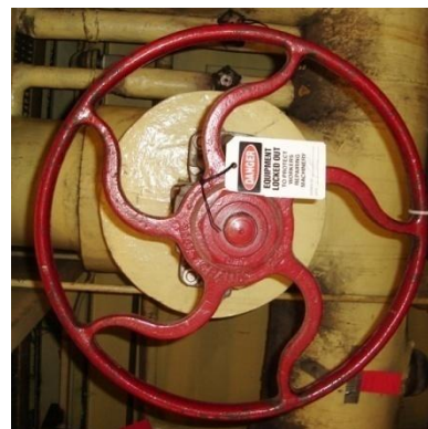
Picture 3: Valve Needs To Be Locked Out, Not Just Tagged
