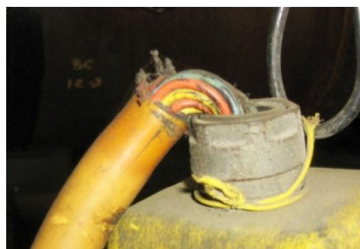
Picture 2: Electric Cord Pulled Away From Mounting
