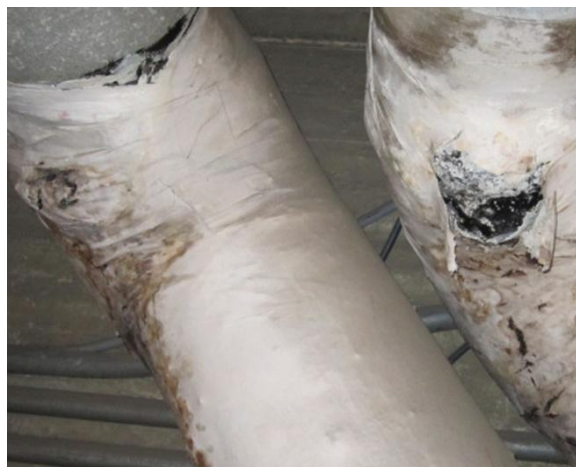
Picture 5: Cloth Pipe Lagging Covers Are Ripped Open Exposing Friable Asbestos Insulation
