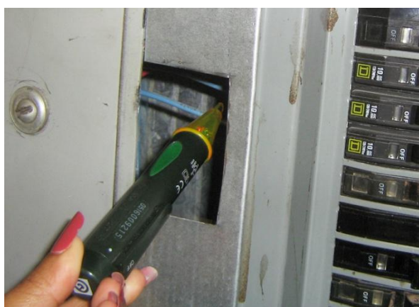
Picture 1: Electrical Box Hole Exposing Energized Contacts
